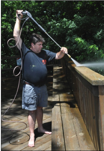
Ed Diehl finishes up the pressure washing of the second deck. Another club will have the pleasure of staining this one.
