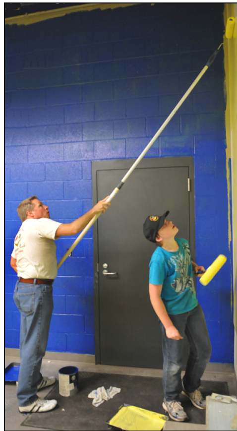
Alan Cowart (L) and Justin Koninsky work on one of the yellow walls.
